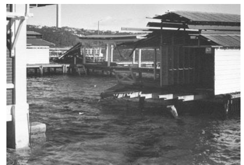
The damaged northern arm of the old baths
